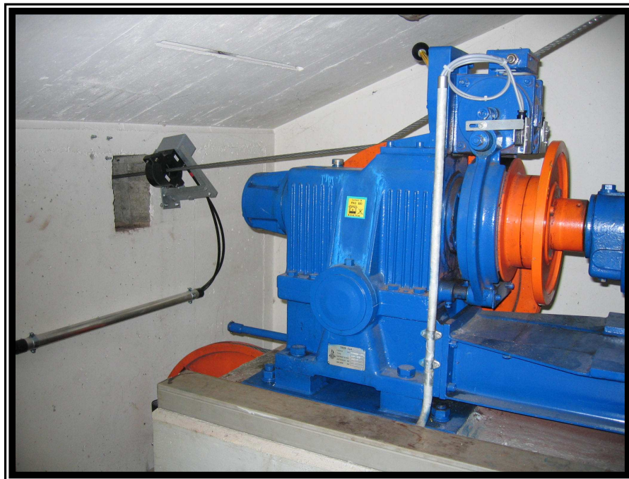
Machine room with transmitter / receiver coils
